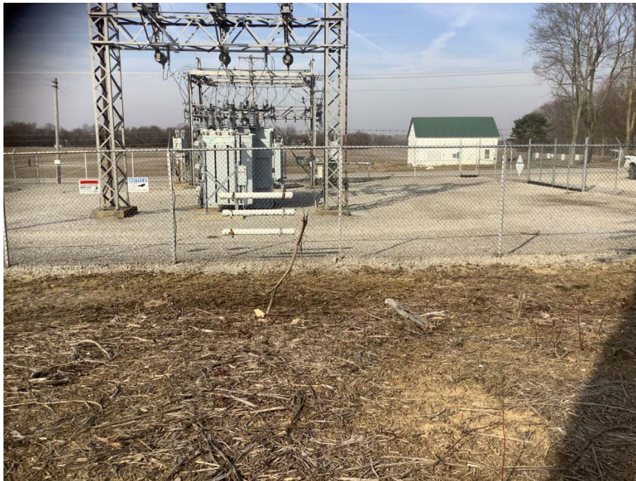
Photo Location 1. Representative view of industrial land (Lott Station) within the Project area. Photograph taken facing west.
